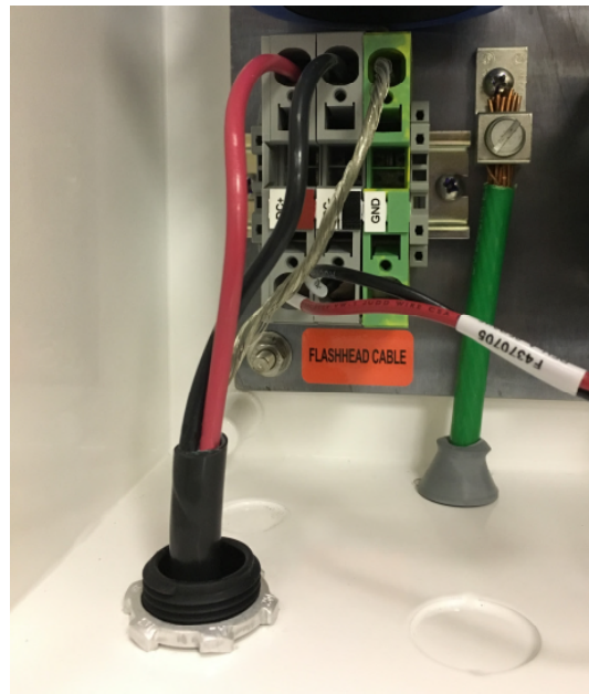
Figure 2-5 – SC 370 Flashhead Cable Connection
